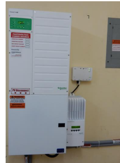
Hybrid Inverter, Charge Controller and Data Logger
