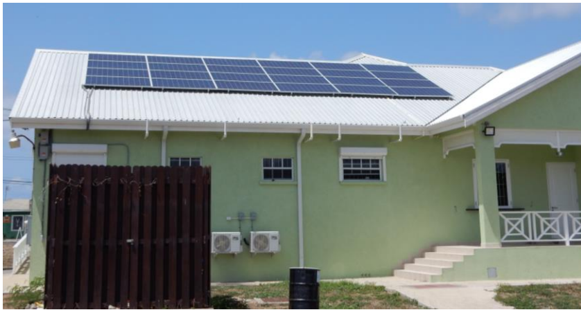
7.5kWp PV System
