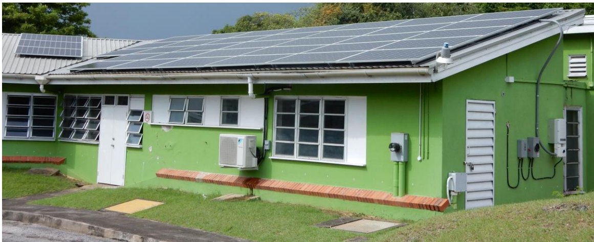
13kWp PV System
