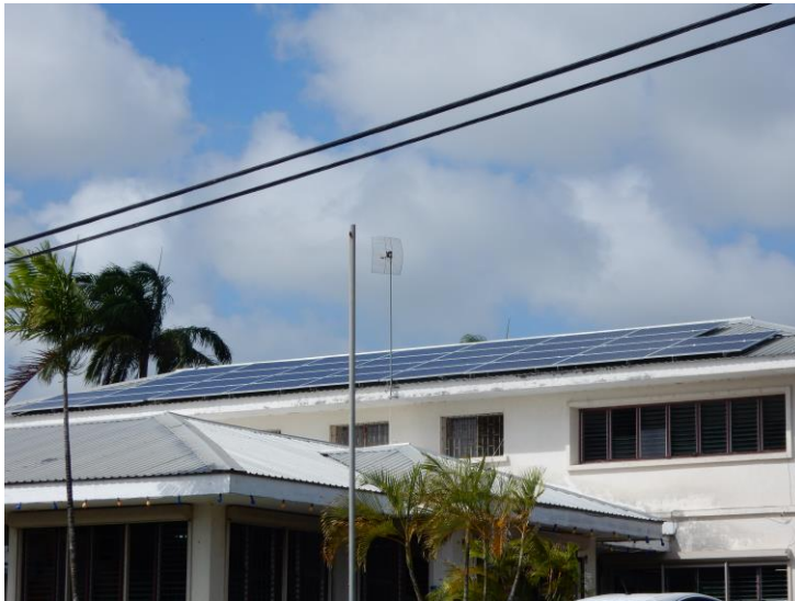
15kWp PV System
